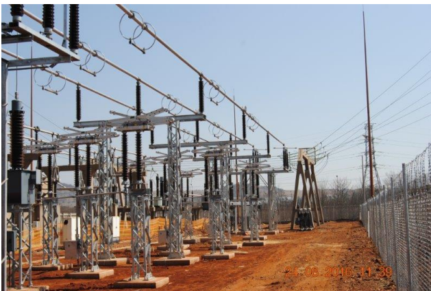
Figure 11: Eldoraigue 132/11kV substation
