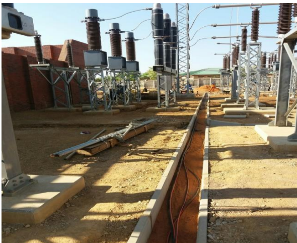
Figure 12: Mamelodi 3, 132/11kV substation
